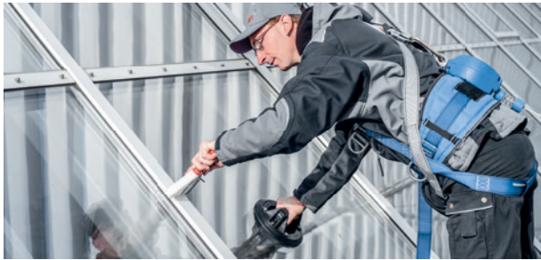
Cleaning of accumulated dirt to ensure correct water drainage (no glass cleaning)
